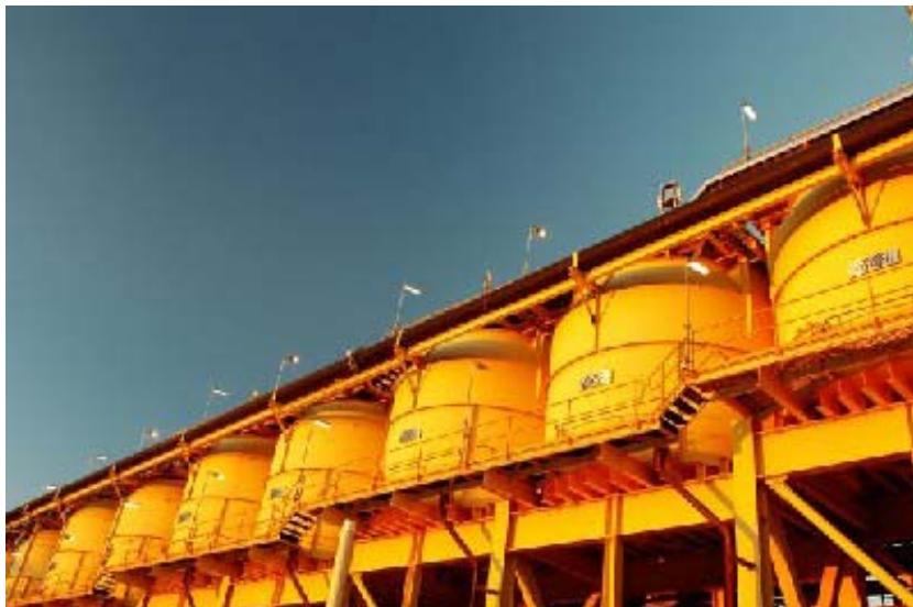
A train of large TankCell® -200 flotation units
