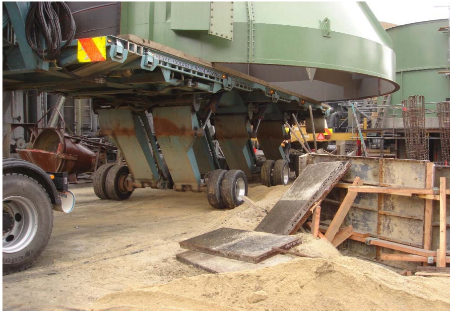
Installation on an exceptionally small existing plant footprint
