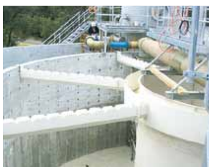
Sludge clarifier, Australia.
