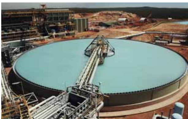
74m tailings thickener, Australia
