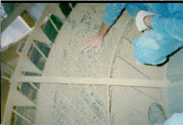
Photograph 9. Primary Air Jig Surface with Revolving Bars and Tailing Launder
