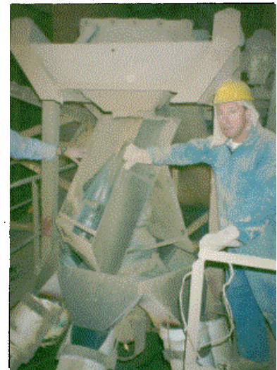
Photograph 7. Rotating Feed Splitter
