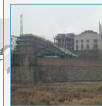
Hunan Zhuye Torch Metals Zinc plant expansion
