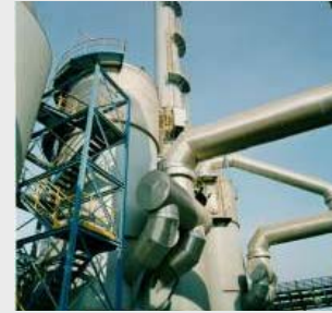
Sulfuric acid plant
